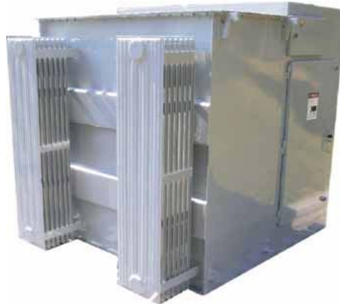
SUB STATION TRANSFORMER
